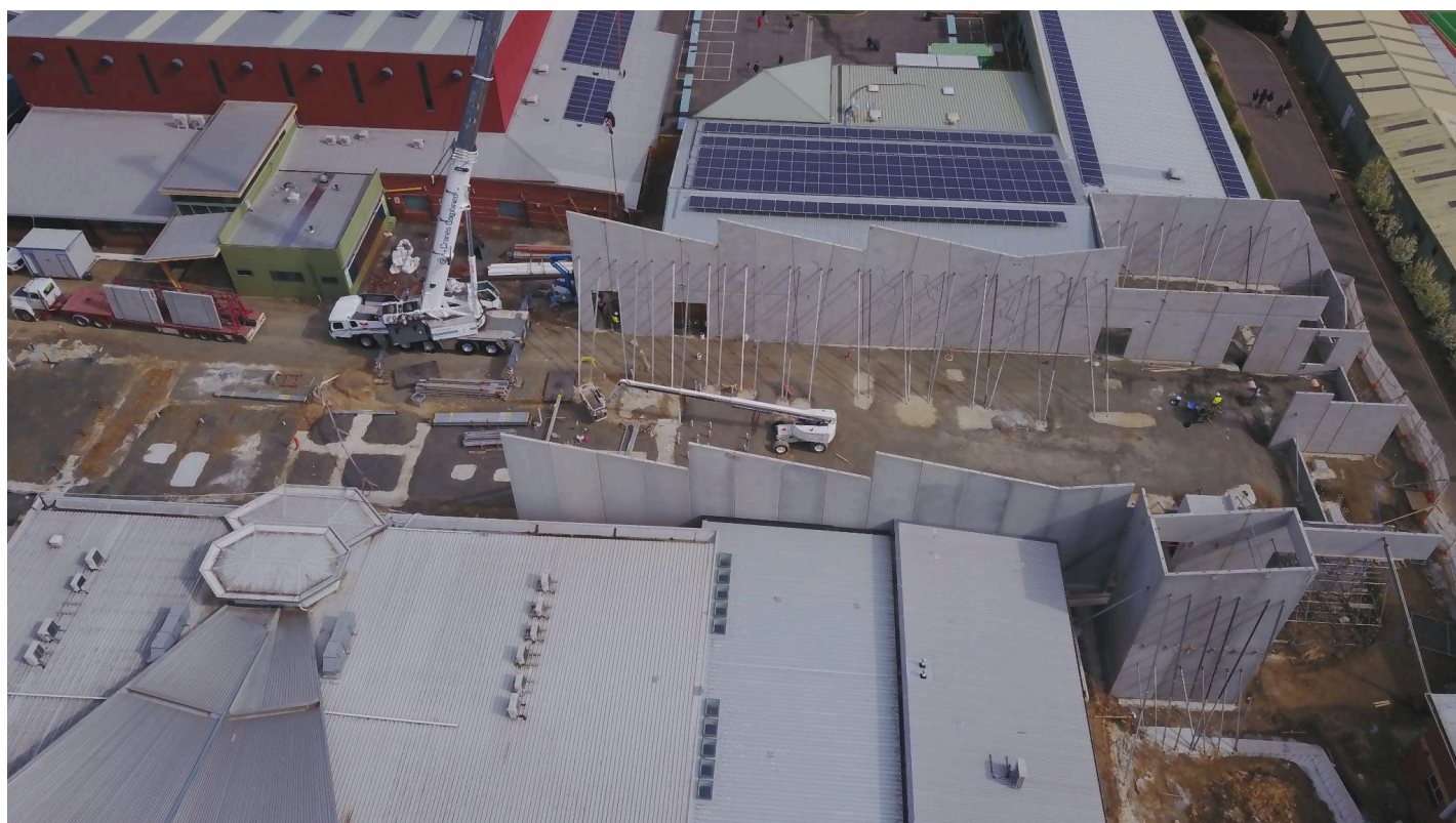
Aerial shot of the site during panel installation, with the Brady Wing at the front of the photo and the Nano Nagle Gym at the top left
